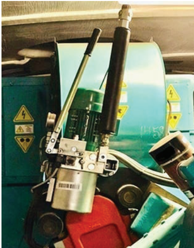
5. A piston accumulator replaced the failed diaphragm accumulator installed on the disk brake assembly shown in Figure 2.
